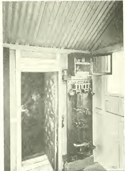
Apparatus in Signal Box with Telephone Cabinet and Operator.
